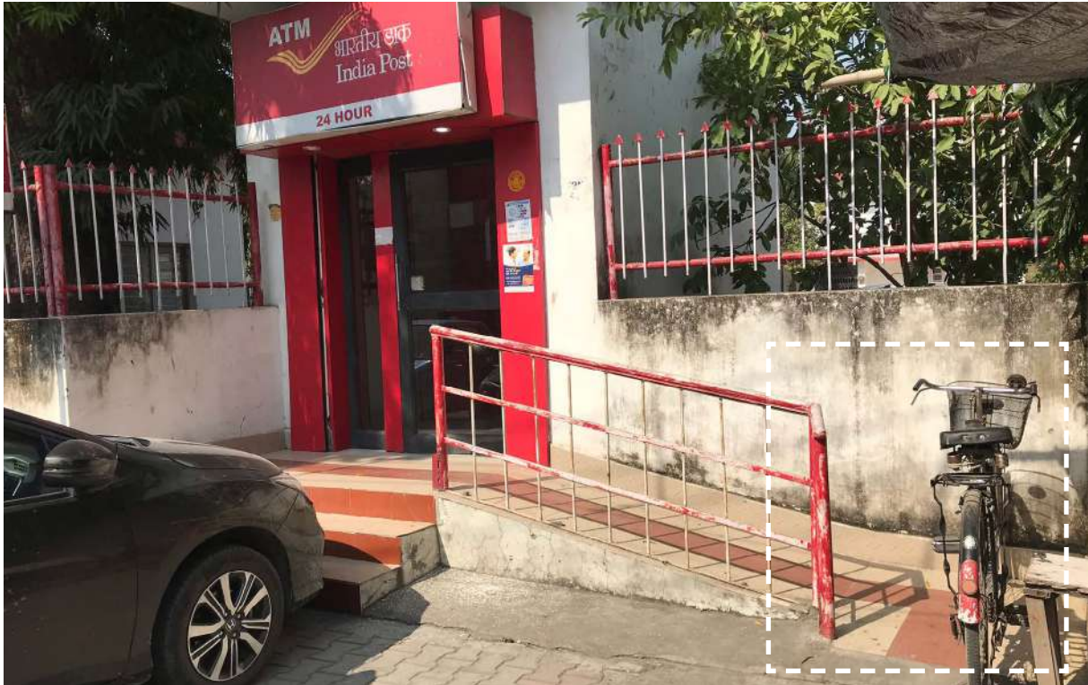
Image 2.24 Improper ramp detailing and management
