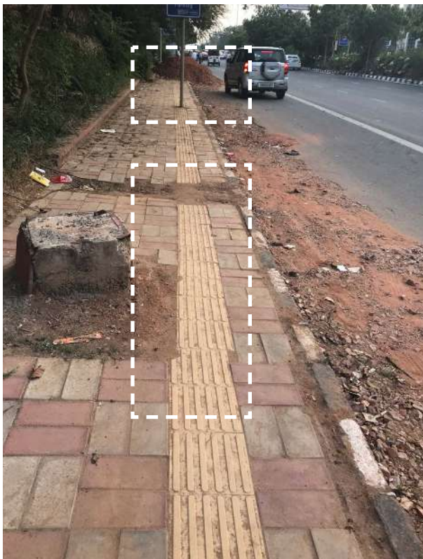
Image 2.19 Poor maintenance of sidewalks and tactile pathways
