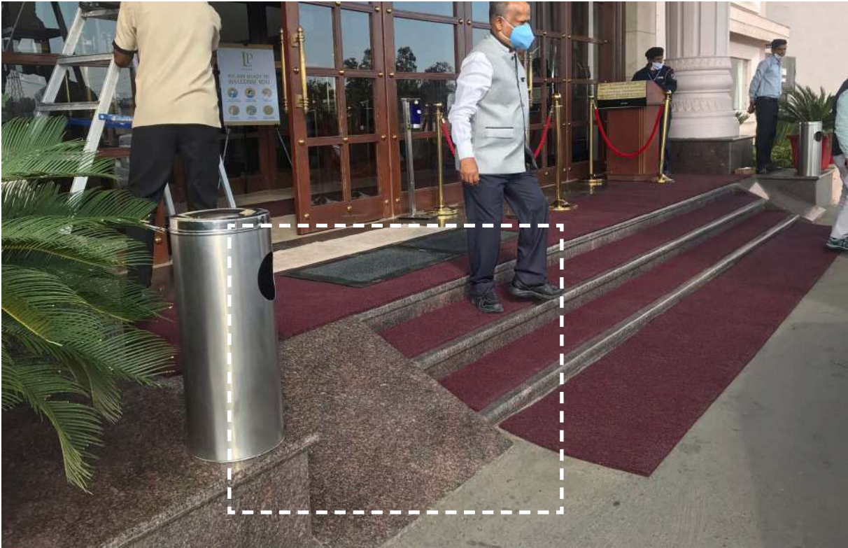
Image 2.7 Improper ramp gradient and slippery floor finish
