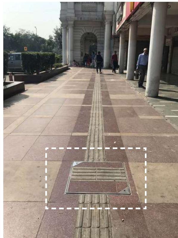
Image 2.20 Inconsistent laying of tactile guiding tiles
