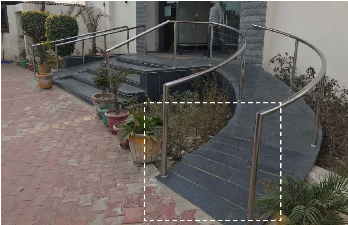
Image 2.9 Curved ramp with improper detailing and design
