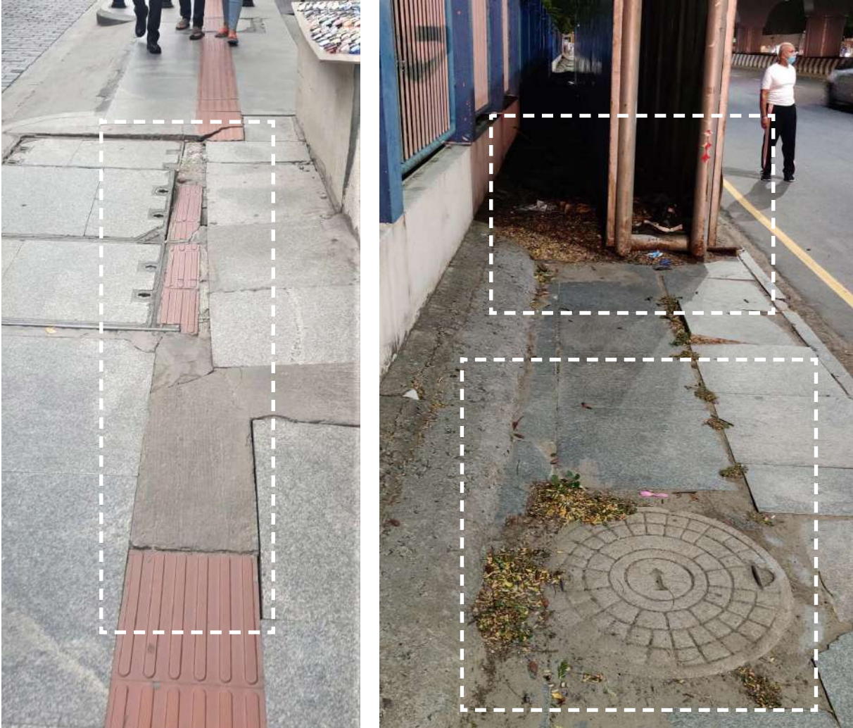
Image 2.17 Inconsistent tactile markings and physical obstructions on sidewalks
