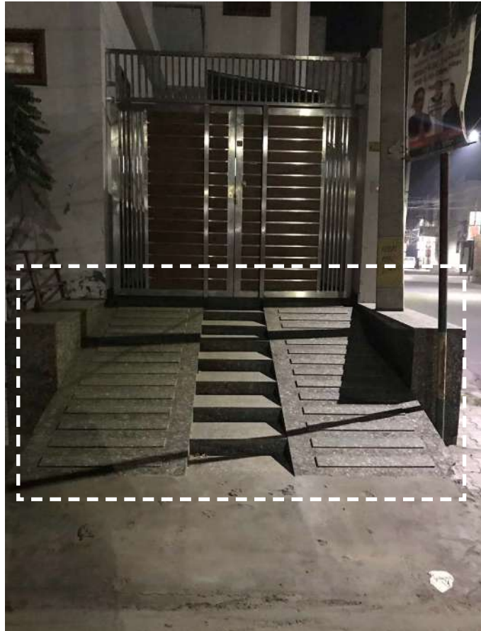
Image 2.14 Improper ramp detailing
