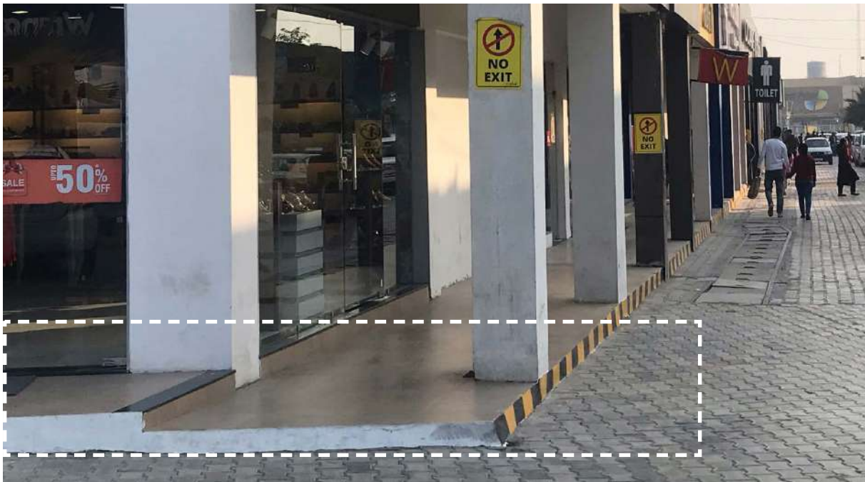
Image 2.15 Improper edge detailing of level change
