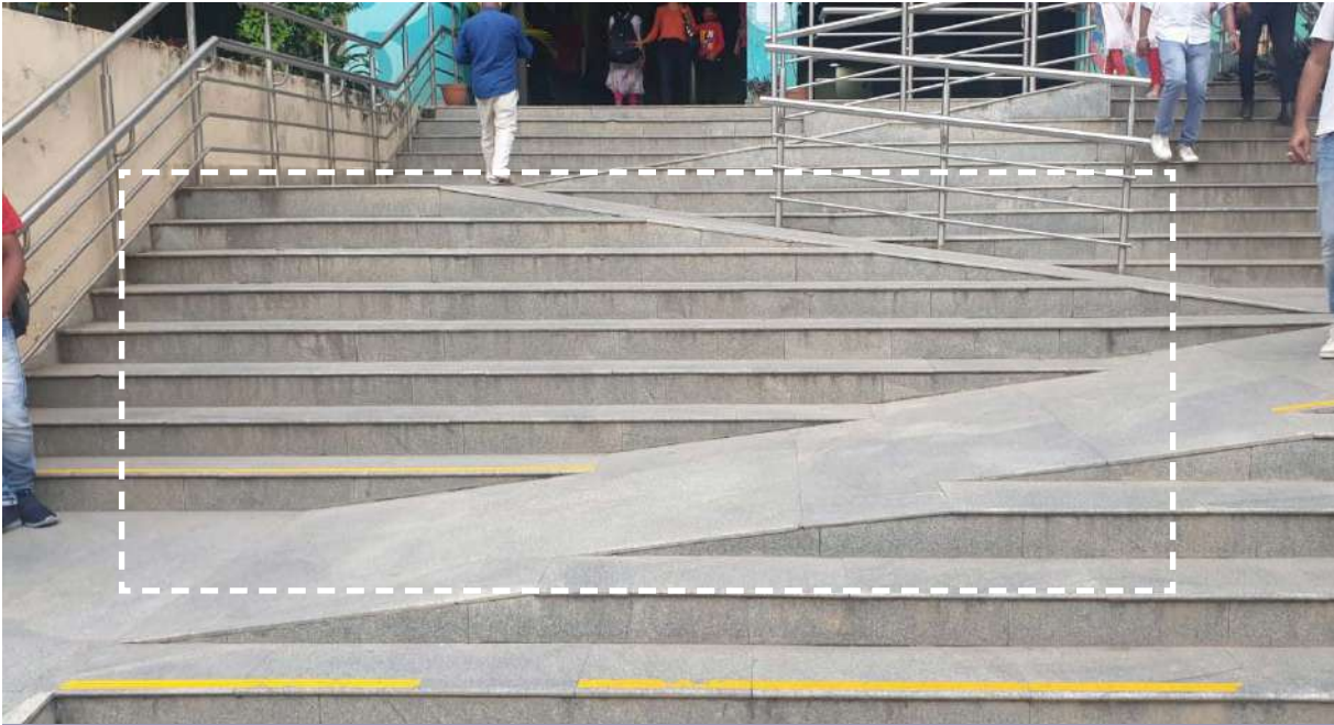
Image 2.11 Inadequate colour contrast
