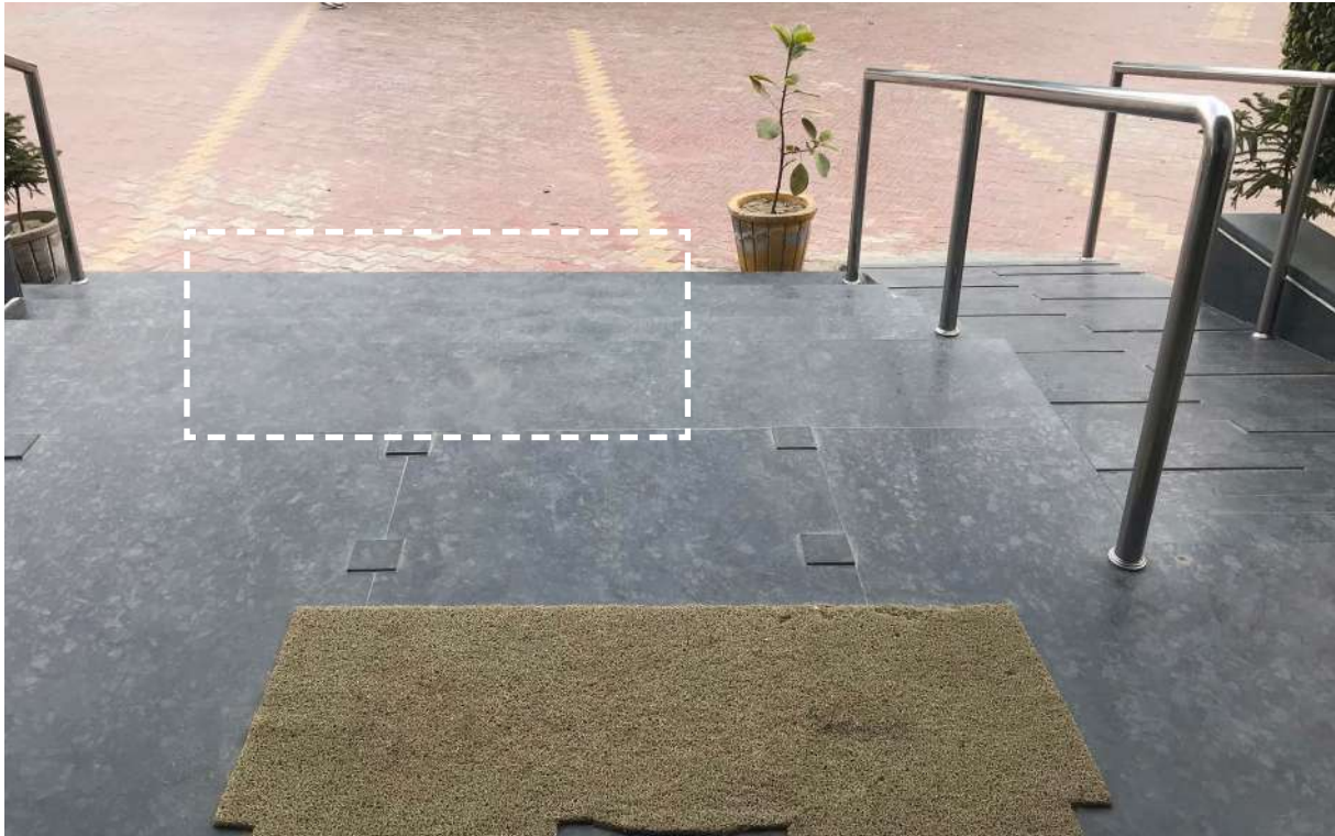
Image 2.18 Poor visual contrast in entrance steps
