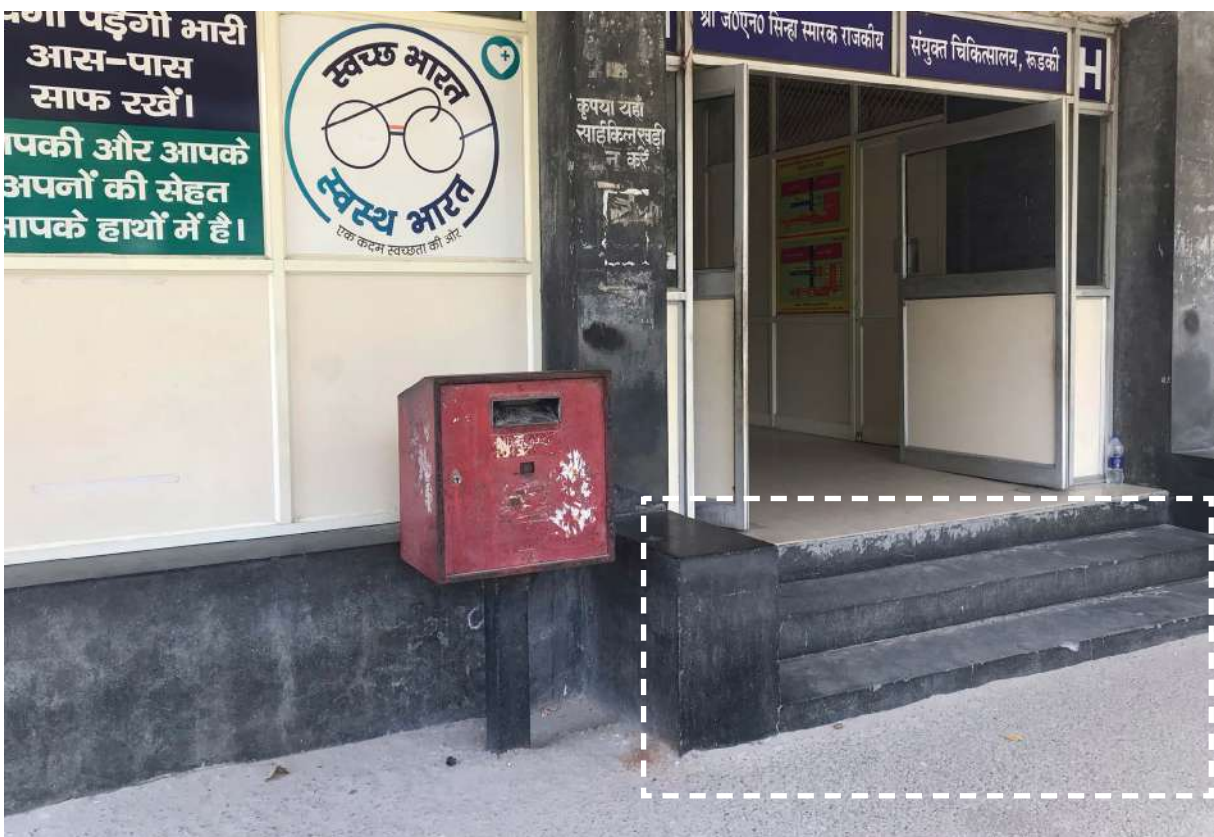
Image 2.6 Inaccessible entrance with inadequate visual contrast in steps
